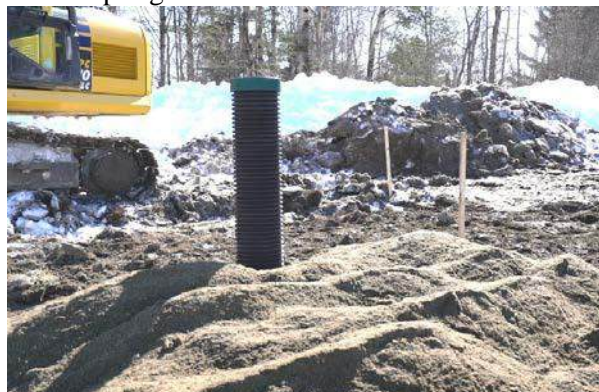
Figure 59. Final installation of the sampling device
