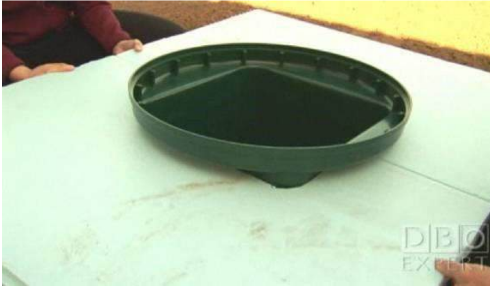
Figure 75. Insulation around a distribution box
