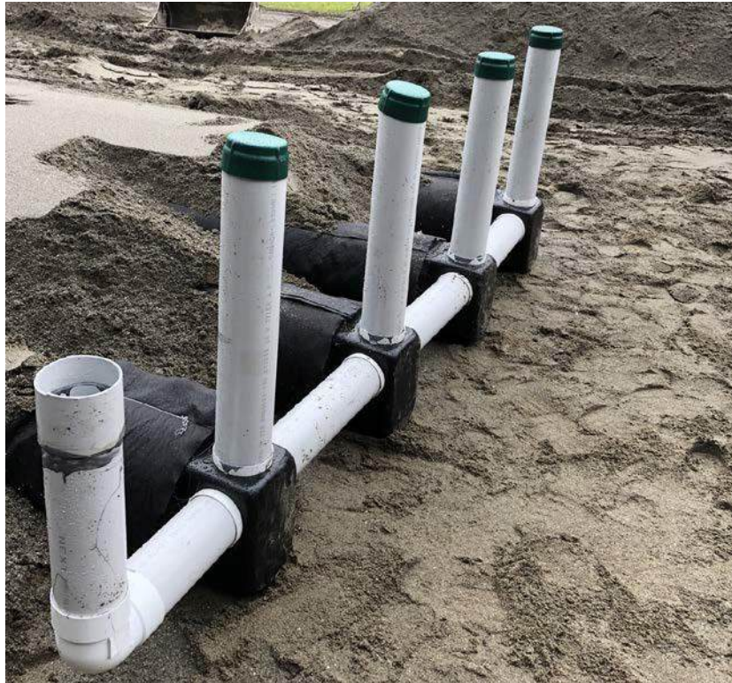
Figure 70. Entry vent on an extremity row
